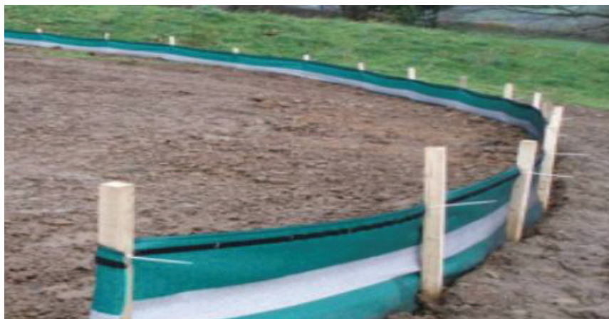
Figure 4.1: Silt Fencing ( www.geosyn.co.uk )
